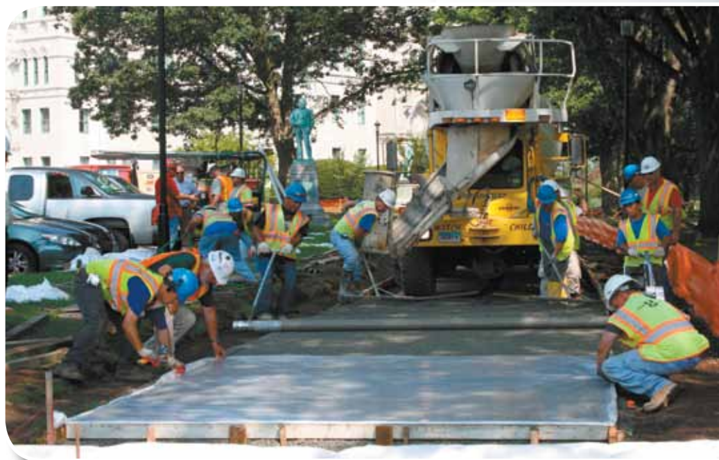
Laydon Industries workers place pervious concrete from Tilcon's Oshkosh truck for Capitols Green Project at Connecticut Capitol in Hartford.
