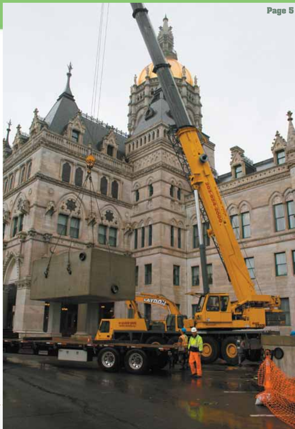
Flanked by Capitol tower, Grove GMK 5120B crane provided by A Quick Pick Crane Service offloads 18-ton cistern from flatbed truck.
