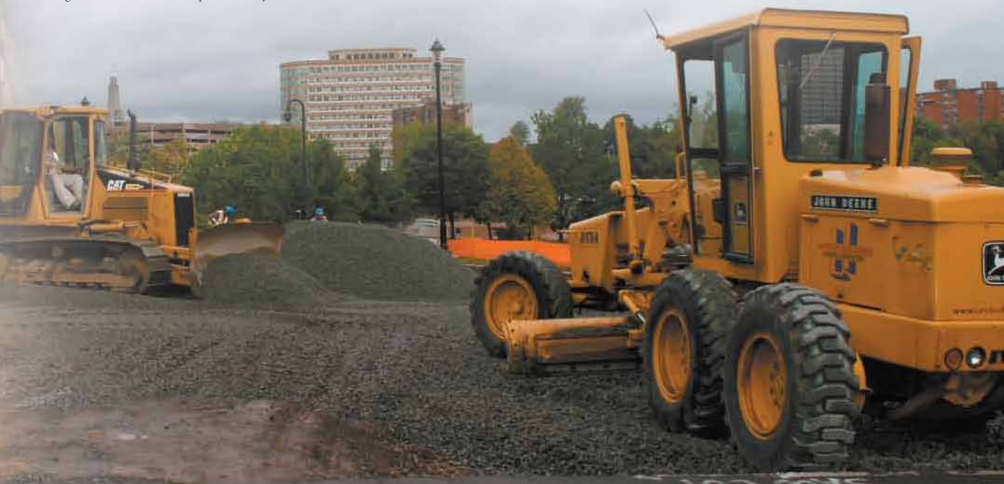
A CAT D5 dozer spreads crushed stone for recharge bed while John Deere 570-A grader finegrades material.
