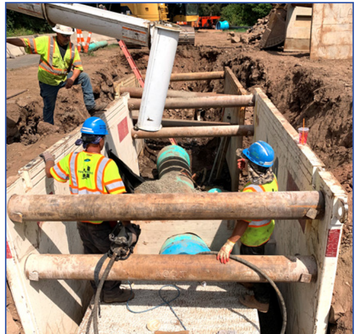
Crews replace the 30" pipe and encase all the fittings with concrete thrust blocks.
