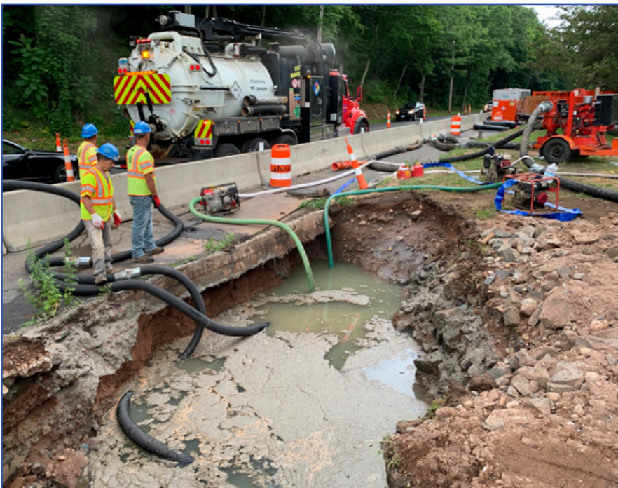
Sewage pipe collapse being drained with a combination of vacuum tanker trucks and a series of 6" and 8" portable pumps.
