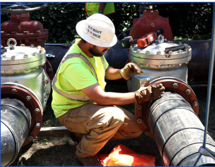
Custom made bypass manifolds using a combination of cast iron, steel, and HDPE components.
